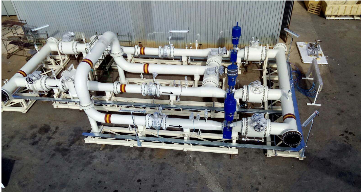
Metering skid with ultrasonic flowmeters – 24 inches 300#RF
