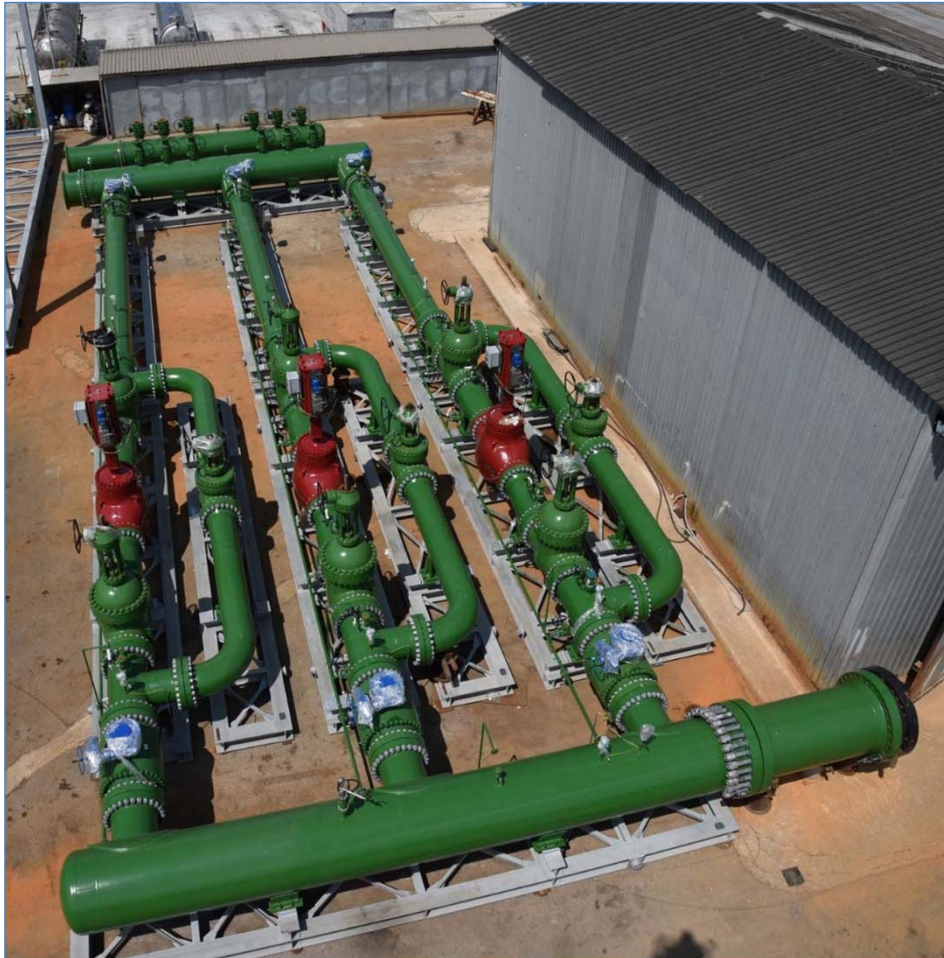
Pressure reduction skid, 48 inches 600#RE, pipe thickness 38mm SCOP – Al-Fao, Iraq
