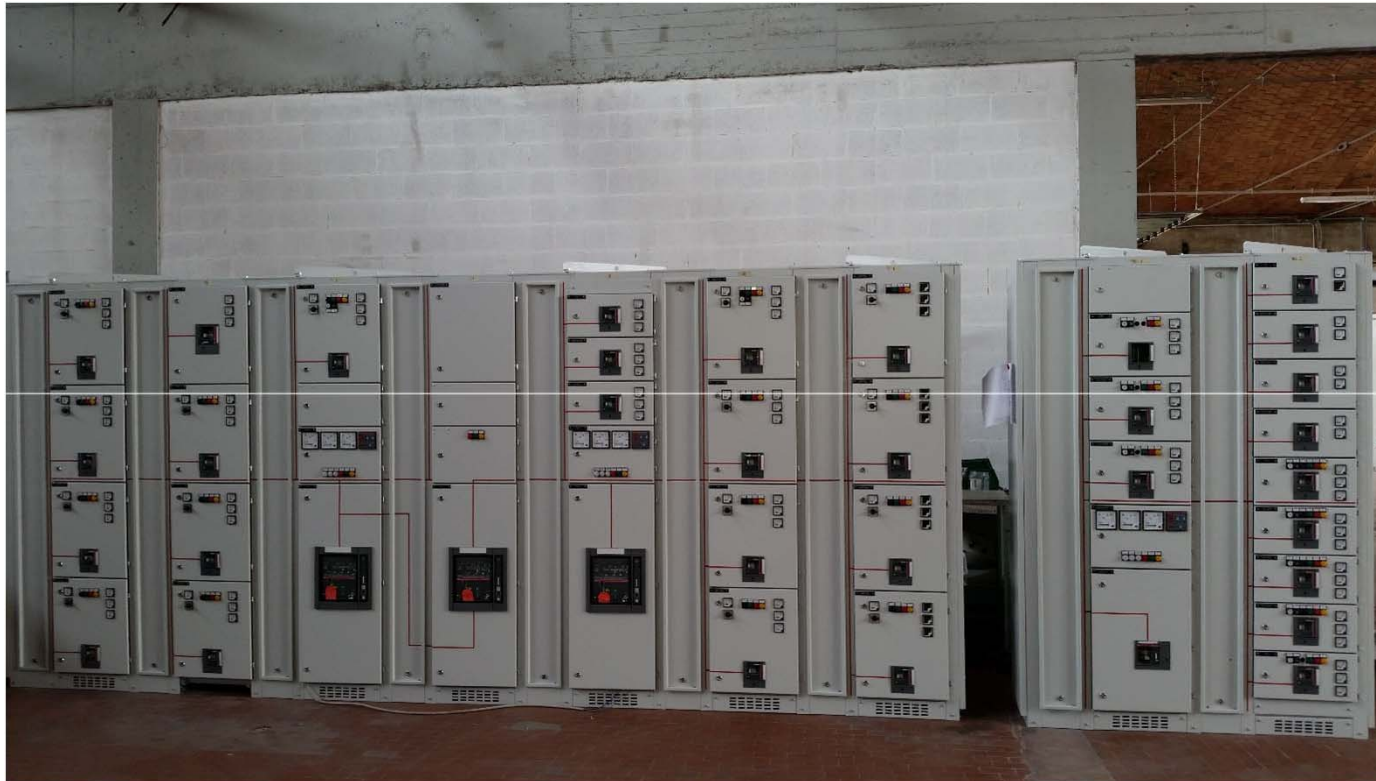
MCC & IYS Boards for LPG Plant
